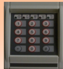
This is an e-key proximity reader. Place your e-key in close proximity to the reader for after hours access.
