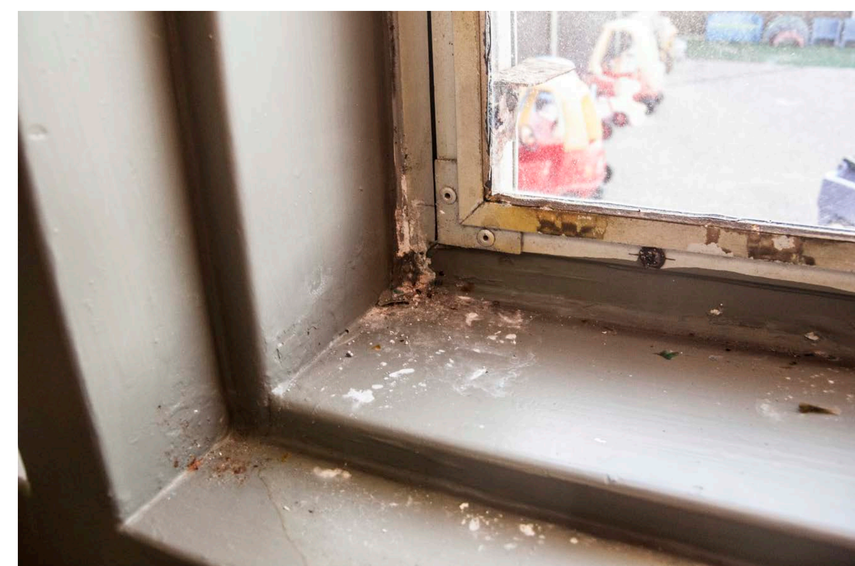
Figure 1. Loma Chica, is apparent on windowsills (shown in the photo) and ceilings. currently a child development center, was built in 1973 for a middle school. Water damage is apparent on windowsills (shown in the photo) and ceilings.
