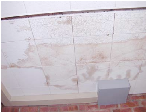
(c) Water damaged ceiling tiles
