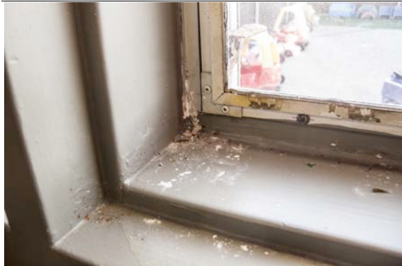
Figure 1. Loma Chica, is apparent on windows sills (shown in the photo) and ceilings. currently a child development center, was built in 1973 for a middle school. Water damage is apparent on windows sills (shown in the photo) and ceilings.
